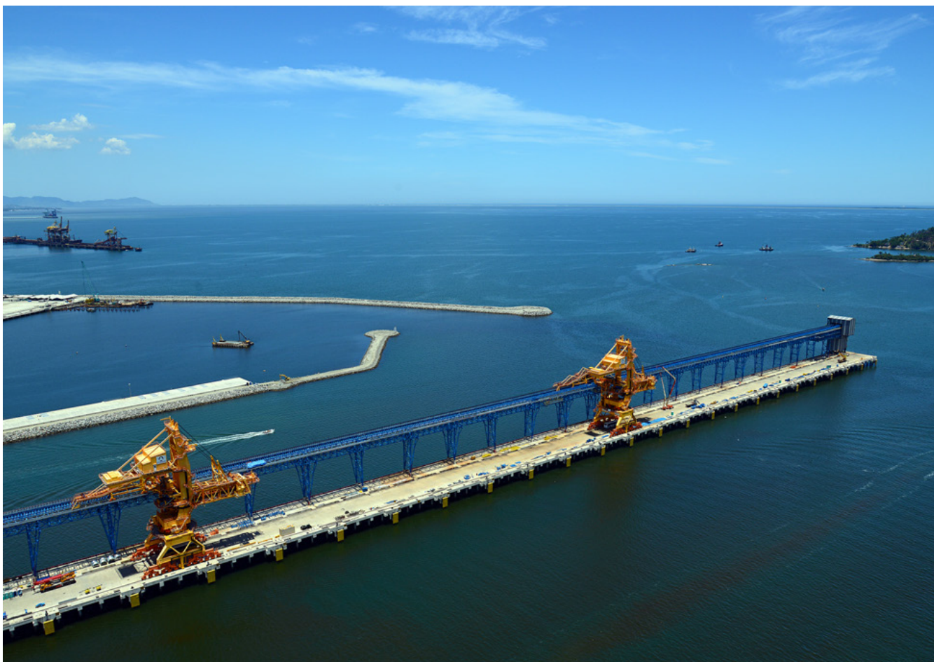
Porto Sudeste iron ore conveyor belt under construction near Rio de Janeiro, Brazil.
