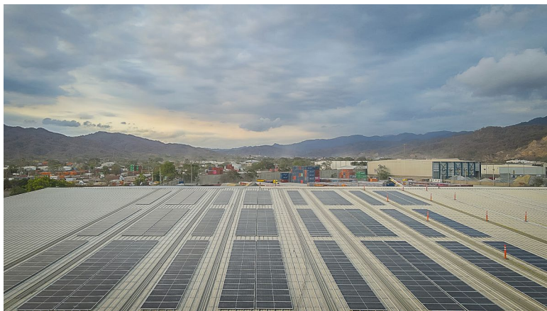
▲ Recently installed solar panels on the roof of Impala Terminals' storage and distribution facility in Manzanillo, Mexico.
